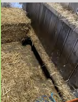
Above: Rabbit Warren entrance compromising shed floor
